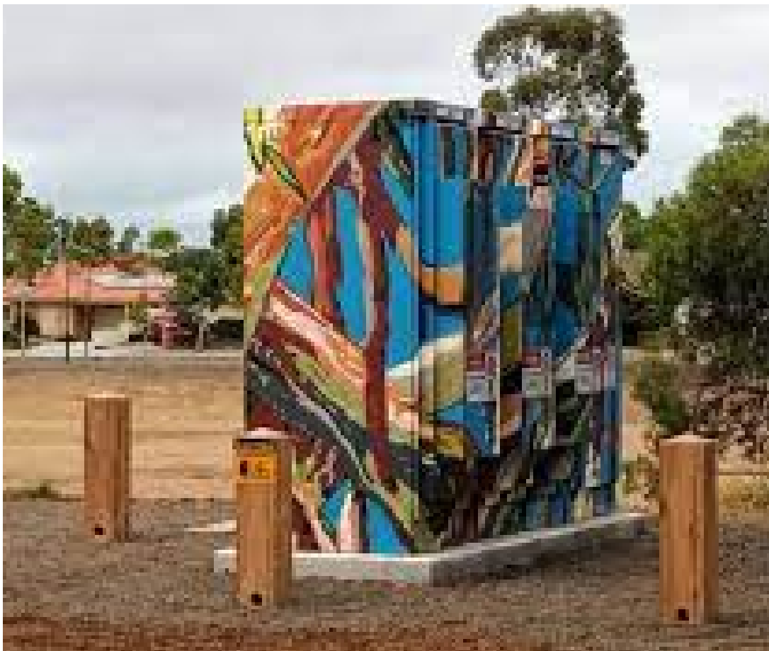
Image of a community battery similar to the Narrabri Community Battery - one of 400 provided across Australia through this funding.
